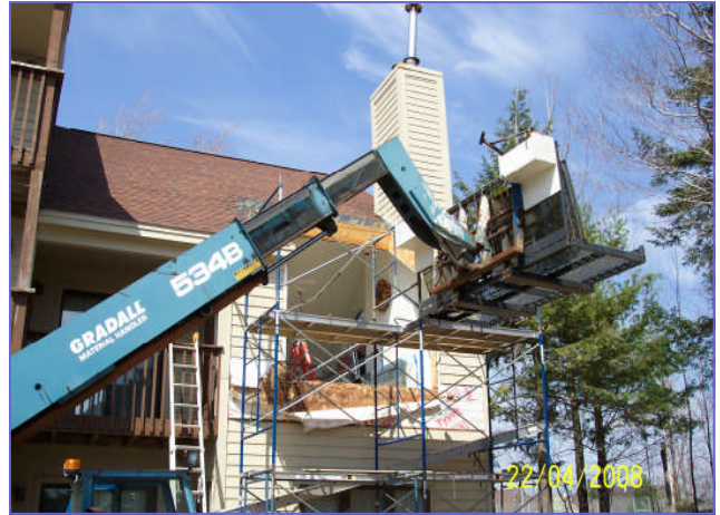
Jeff Milligan and Associates install sky light replacements and work on building repairs
